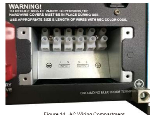
Figure 14 AC Wiring Compartment
